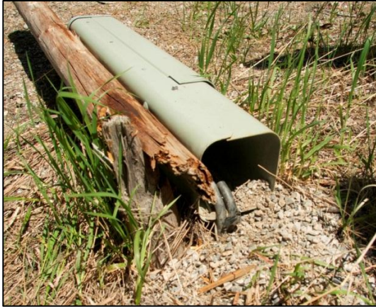
Dark fiber lies unconnected on the side of the road within the borders of the Colville Reservation. For Tribal members, the long stretch of dark fiber running within a roadside ditch – displayed on maps as actively supporting deployed telecommunication services – was a great source of frustration.
